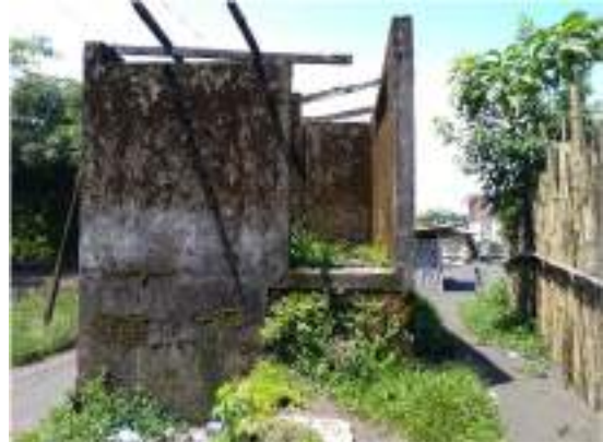
Lone Delapitated Idenau Public Toilet
