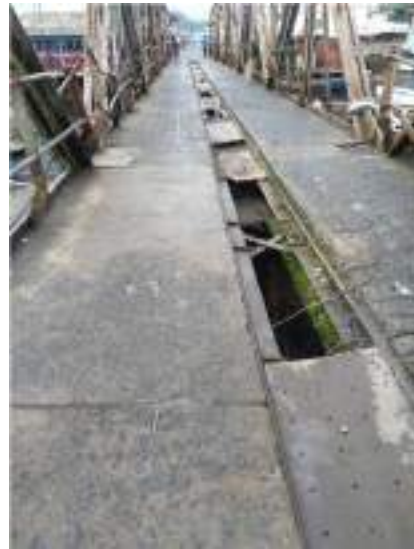
Delapidated Idenau Main Bridge
