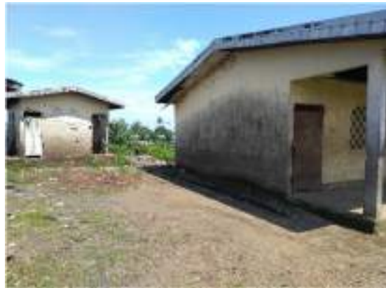
Delapitated School Toilet
