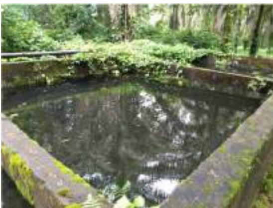
Insanitary Main Water Supply Tank of Idenau
